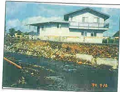
Streambank Erosion caused by the 1994 flooding of Waiakea Stream.
