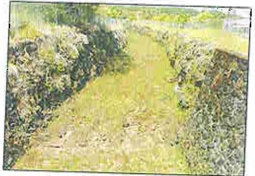
Portion of the Akolea diversion installed to protect homes in the Ainako subdivision.
