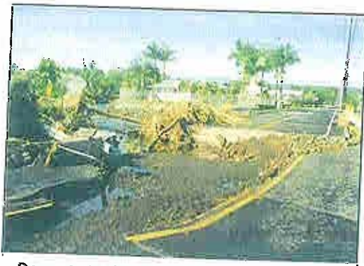
Damage to the Kawailani bridge from the November 2000 flooding of Waiakea Stream.
